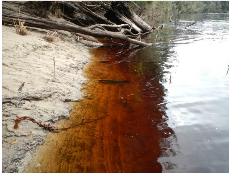
Figure 3-7: Erosion pin site 4A downstream of Denison River confluence showing inundation of erosion pins.
