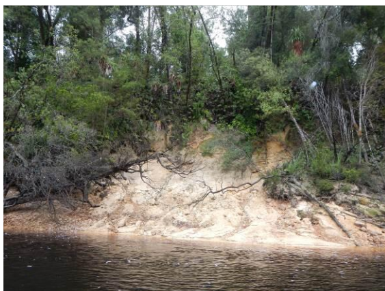
Figure 3-23: Seepage slumping at landslip site in zone 2. Site is located on the left bank, d/s of erosion pin site 2A.
