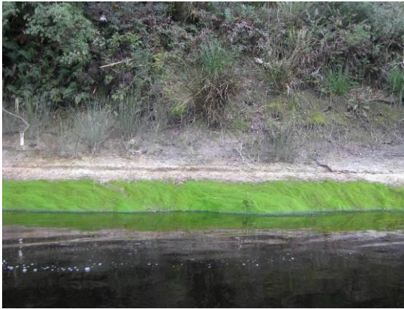
Figure 3-15: Algae on bank toe in erosion pin site 2C (zone 2), with increased vegetation upslope.
