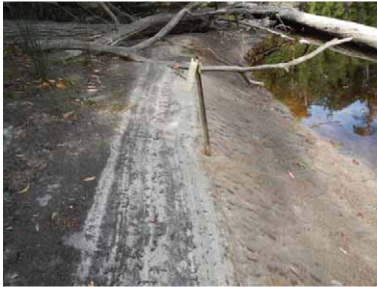
Photo 4-14 Break in slope at ~1–2 turbine discharge level, algal deposit upslope of break in slope, and mud veneers and organic debris on bank face at erosion pin site 2D, February 2012
