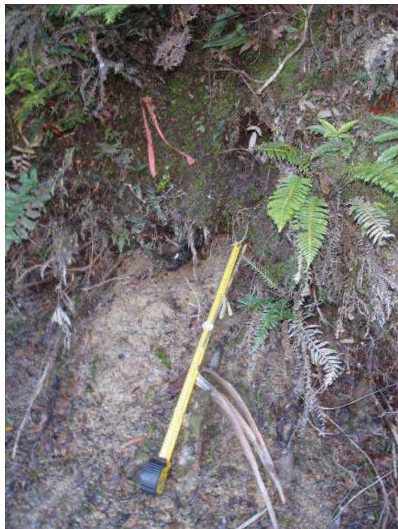
Photo 4-4 Dried sediment flow at erosion pin site 2C indicative of past seepage erosion, probably during prolonged high flows during winter
