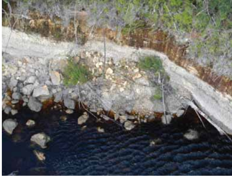
Photo 4-16 Aerial view of recent bank failure in the Albert River, left bank upstream from Gordon confluence
