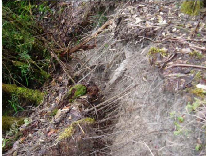
Photo 4.1. Scarp created by bank collapse at site site 5A.
