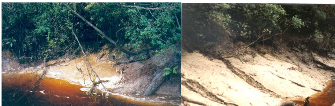
Photo 3.8. Active seepage erosion (water and sediment exiting bank) following power station shut-down (left) leads to sediment flows (right) on alluvial banks in zone 2.
