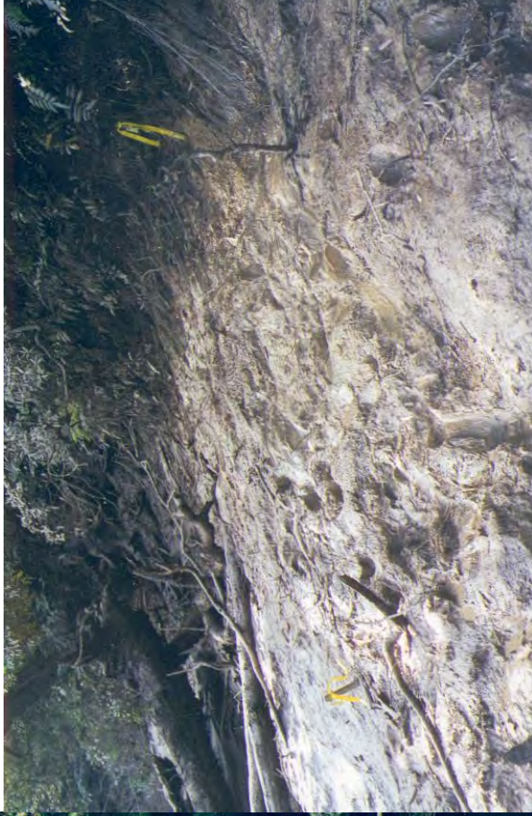
Photo 66. Downslope movement of erosion pin in Zone 2
