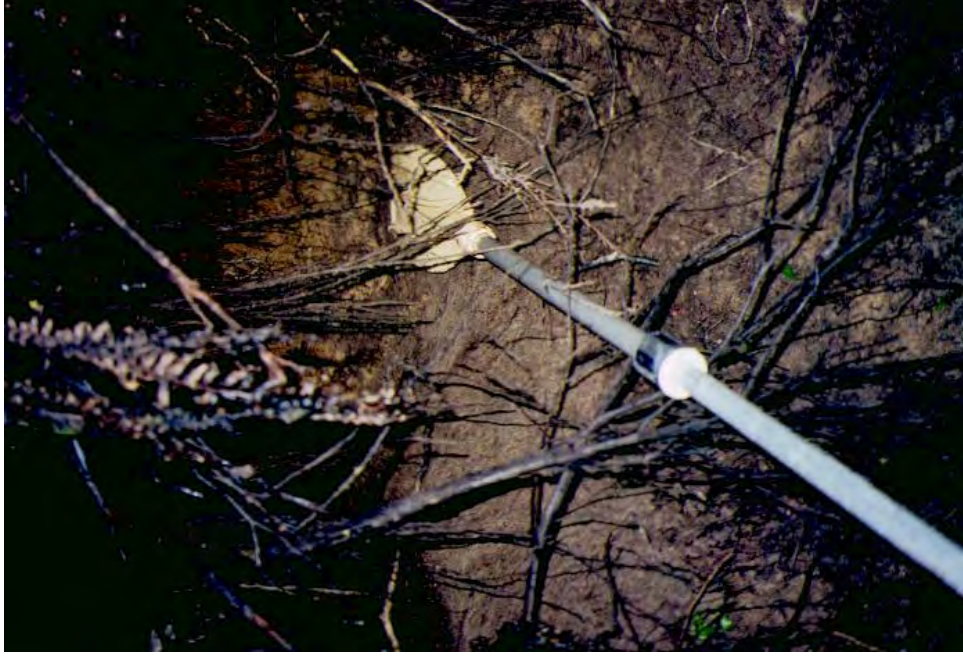
Photo 32. Large void in Franklin River
