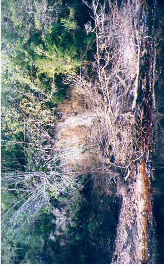
Photo 13. Slip in vertical cobble bank in Zone1 (note weathered appearance of cobbles to left of slip)
