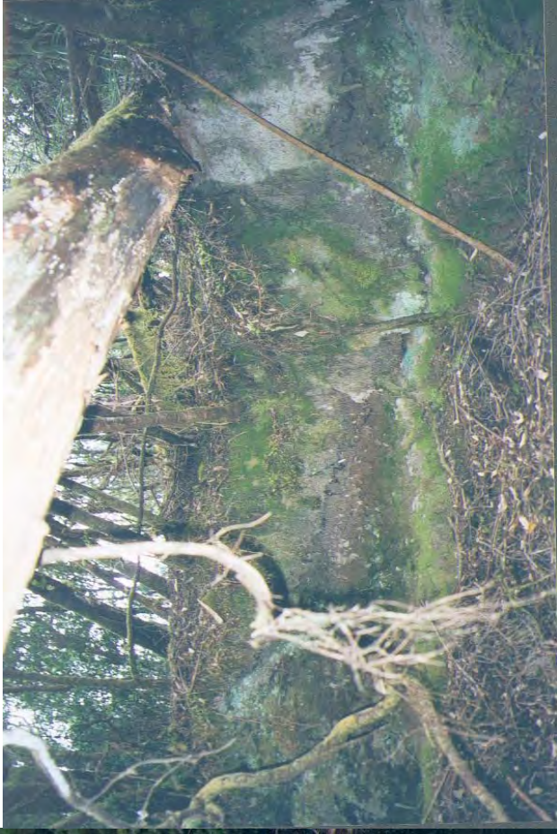
Photo 36. Undercutting of river bank on Gordon River approximately 7 m above present high water level
