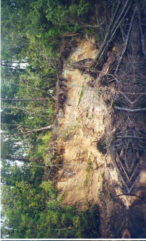
Photo 21. Land slip in cobble unit in Zone 2
