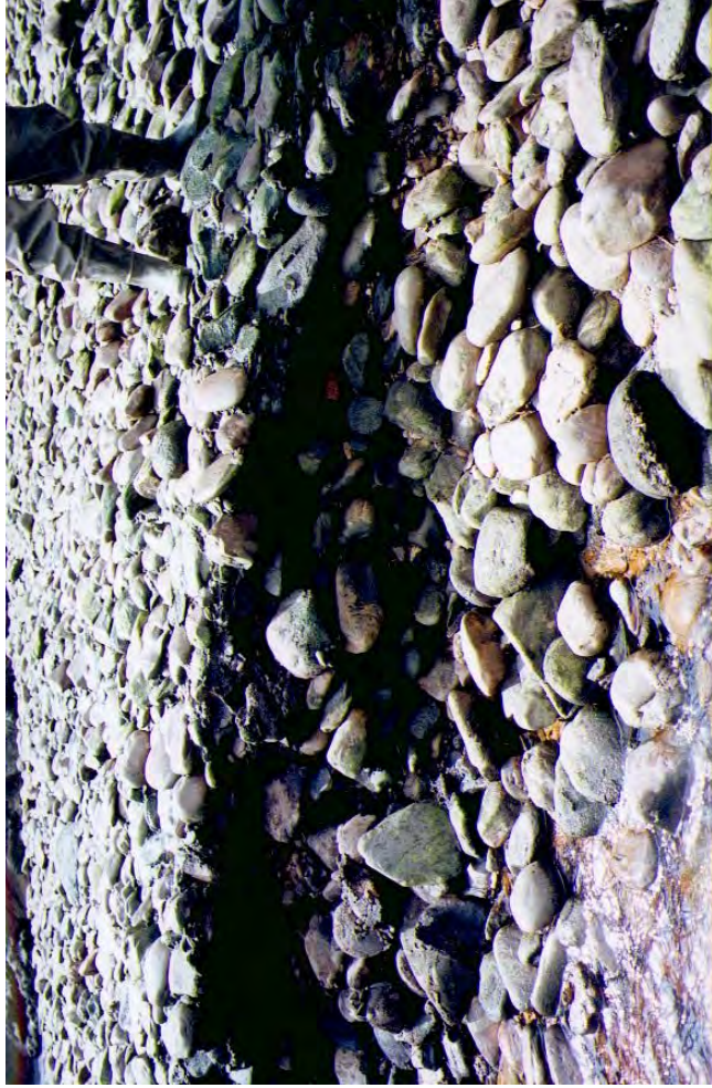
Photo 41. Undermining of cemented surface
