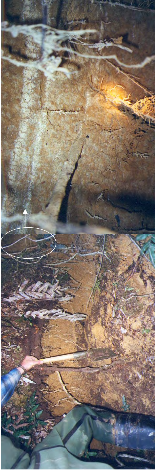
Photo 57a&b. Foam lines indicating high water level on wall of void
