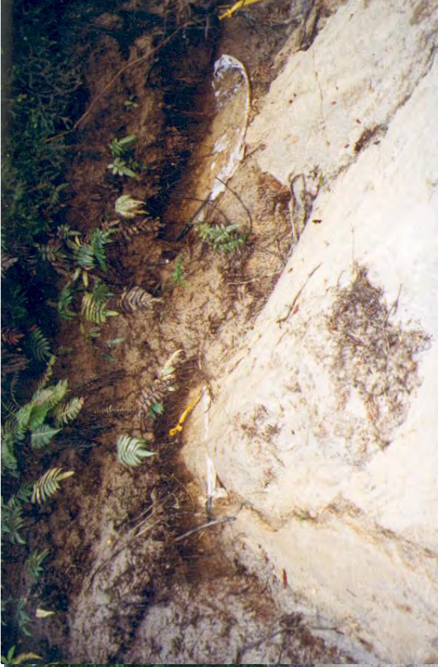
Photo 61. Seepage erosion features in the Gordon River
