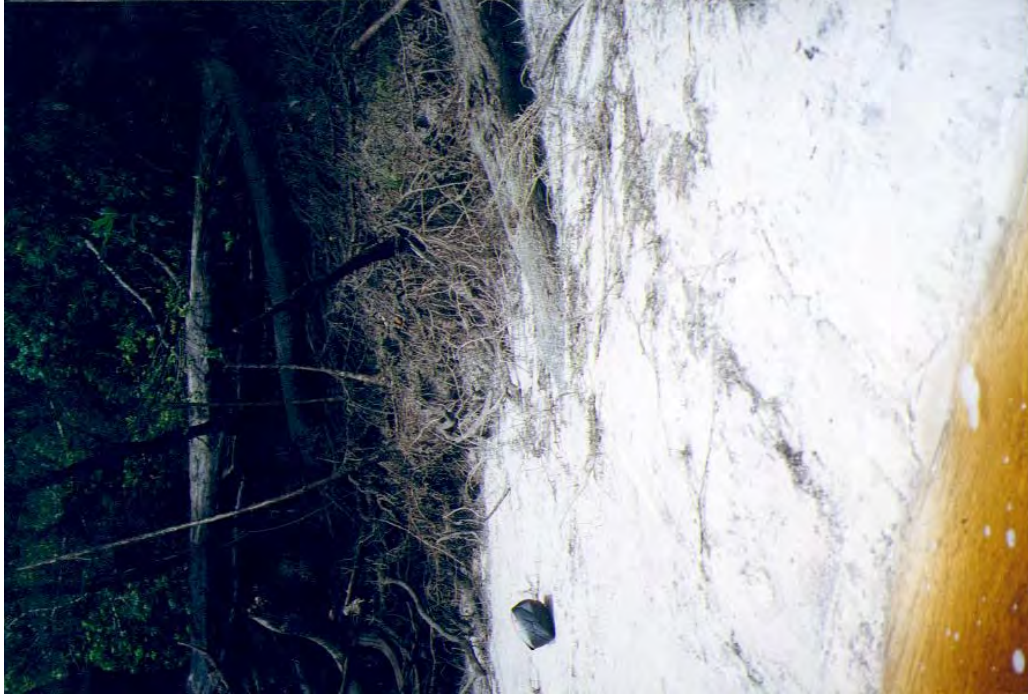
Photo 62 Exposed tree roots due to scour
