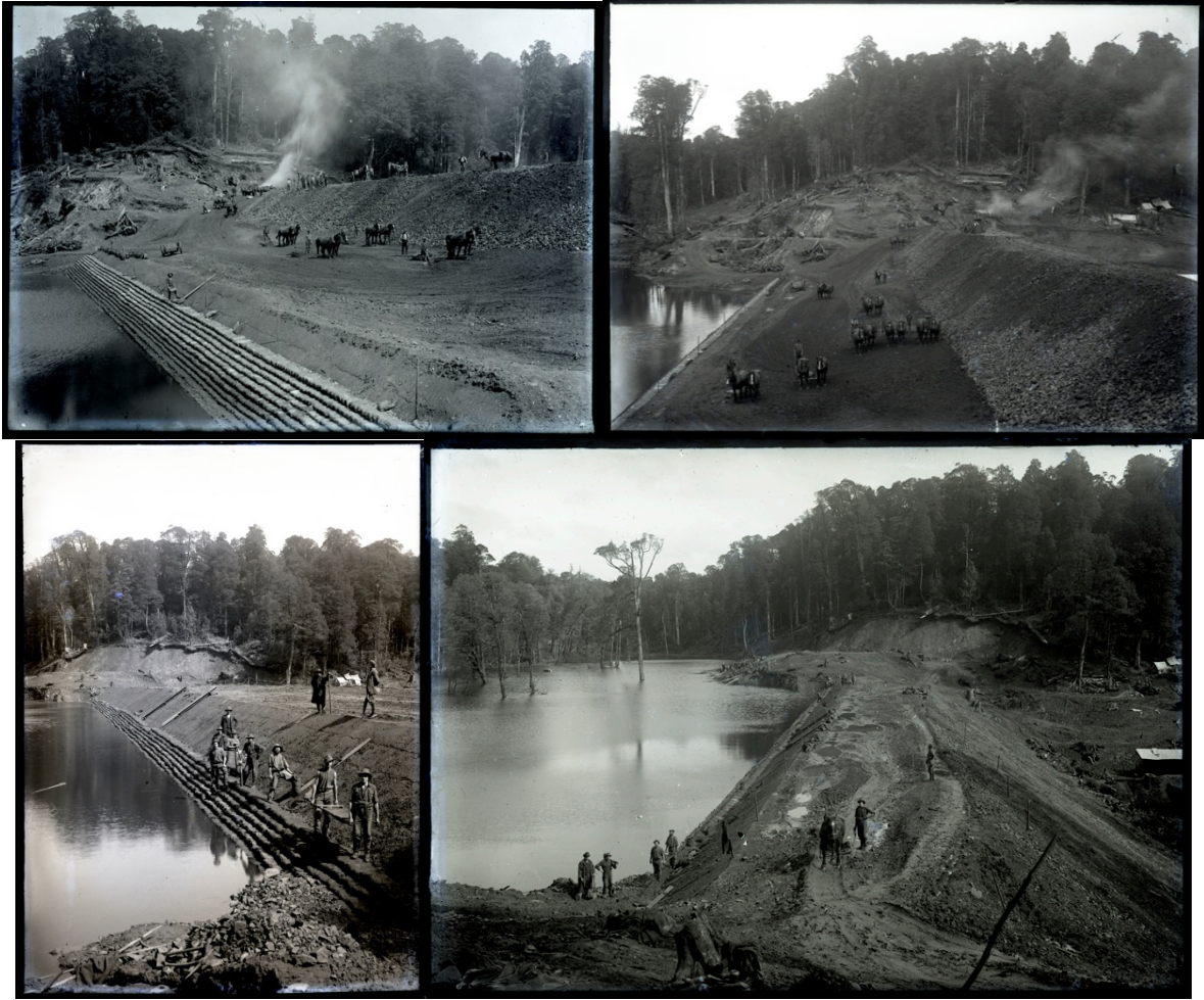
Construction of the Magnet no.2 Dam on Magnet Creek, 1918, for the Magnet Silver Mining Company. This earthfill dam, like the Waratah Dam, was built to provide extra water for a mine's hydro-electric power plant.
