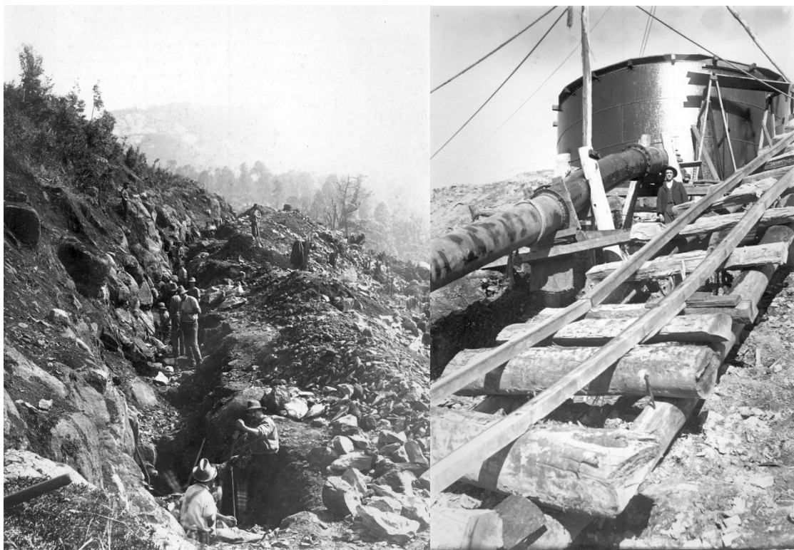
(Left) The laborious job of water race construction around the slopes of Mount Bischoff for the Power Station. Probably a JH Robinson photo, from the Weekly Courier , 6 June 1906, p.22. (Right) The Black Tank, showing the pipeline and haulage way down to the Power Station. Photo courtesy of the Waratah Museum.
