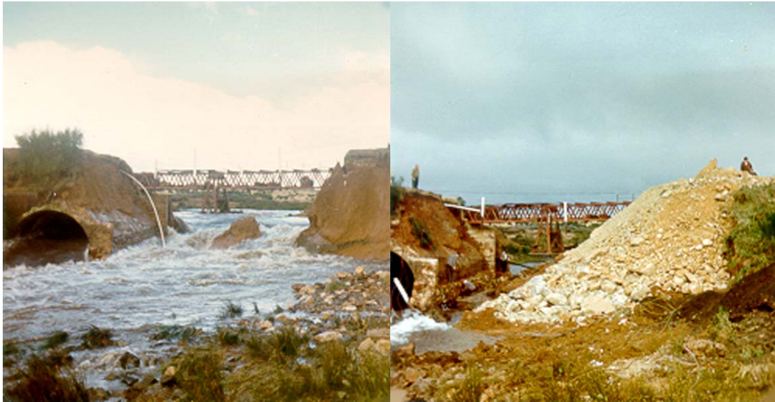
The aftermath of the Waratah Dam burst in May 1975, with the Smith Street road bridge being destroyed. Photos PH30-1-4875 and PH30-1-4876 courtesy of LINC Tasmania.
