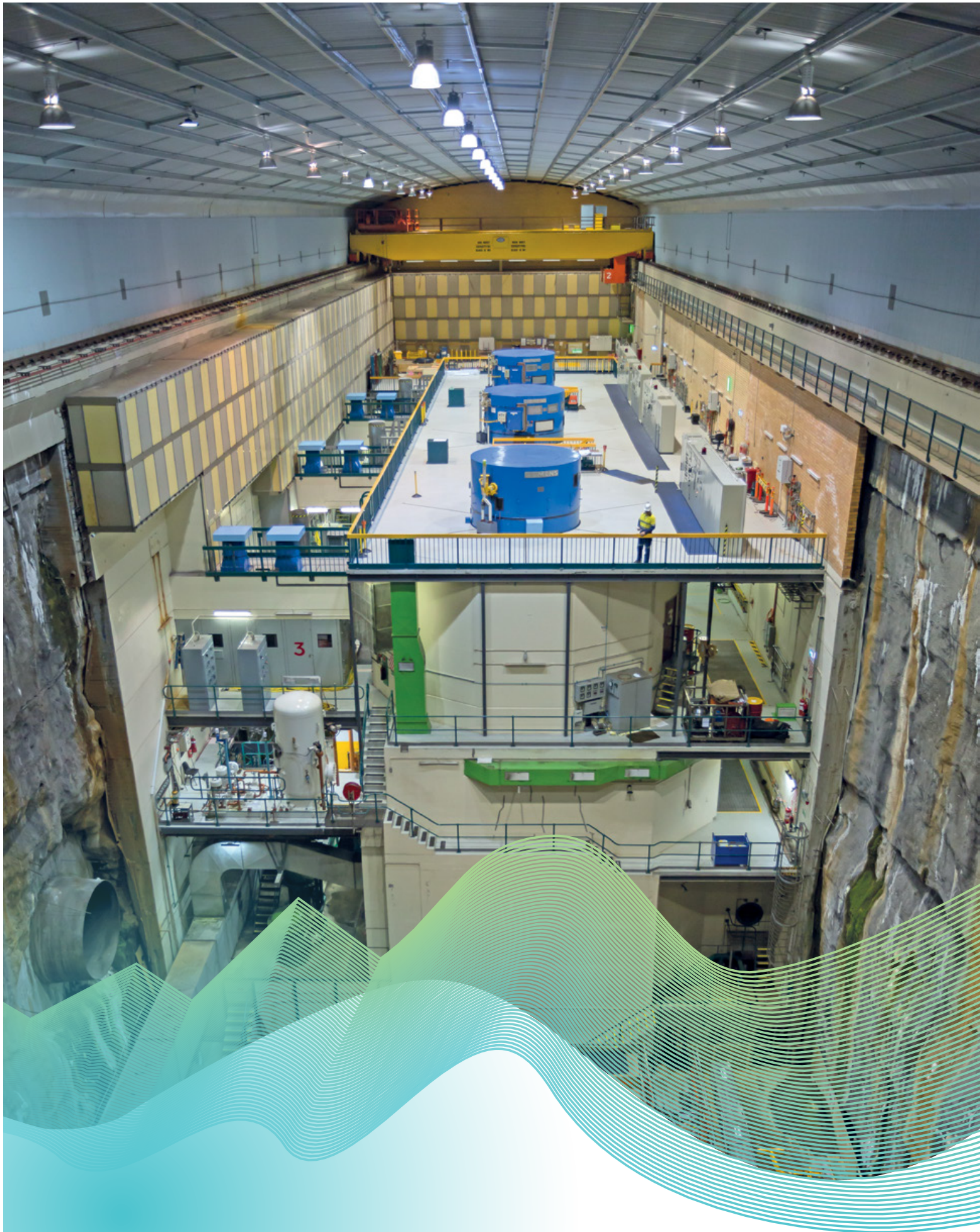
Above: Gordon Power Station at Strathgordon
