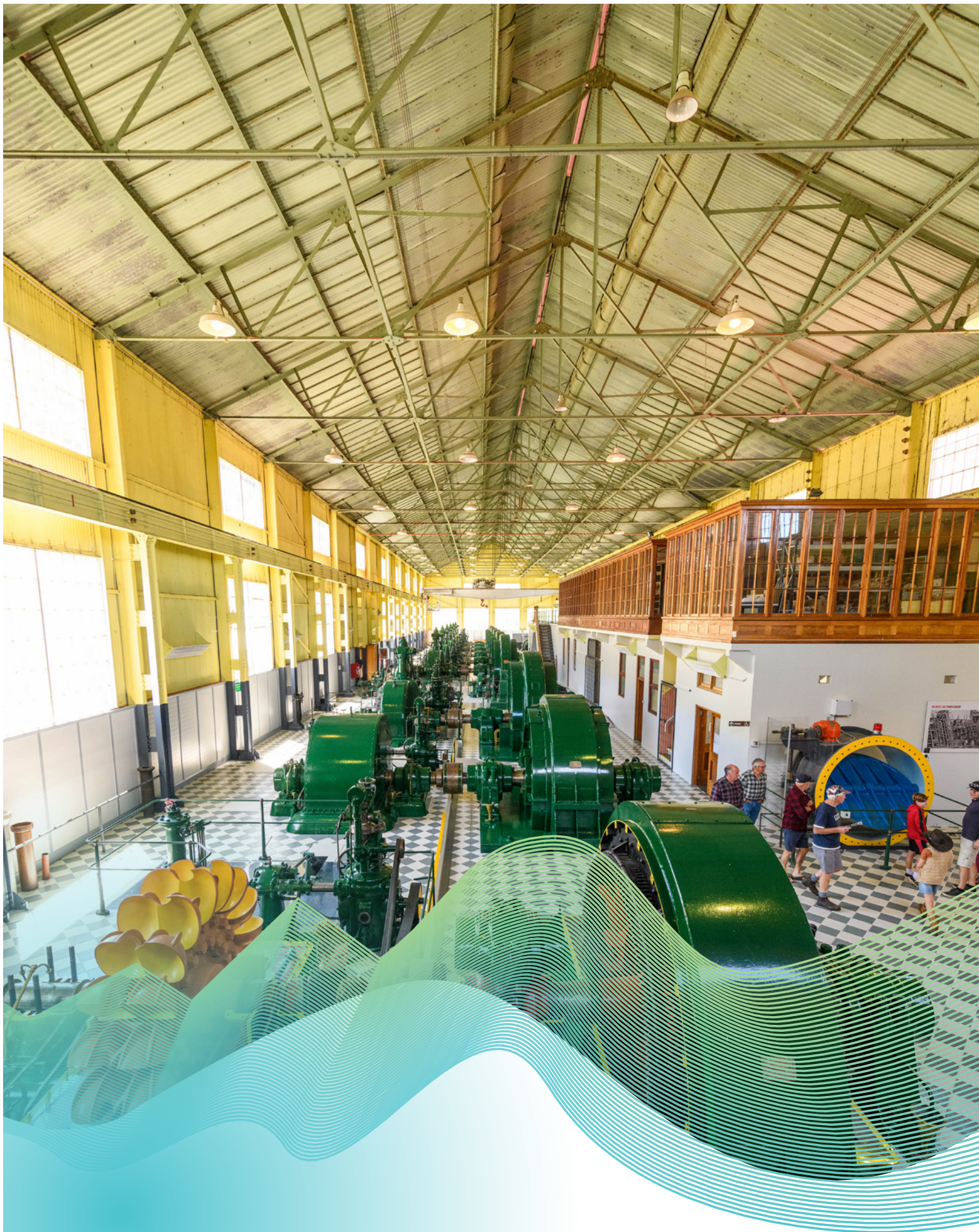
Above: Waddamana was Hydro Tasmania's first power station and now as a heritage site, it welcomes more than 7,000 visitors annually
