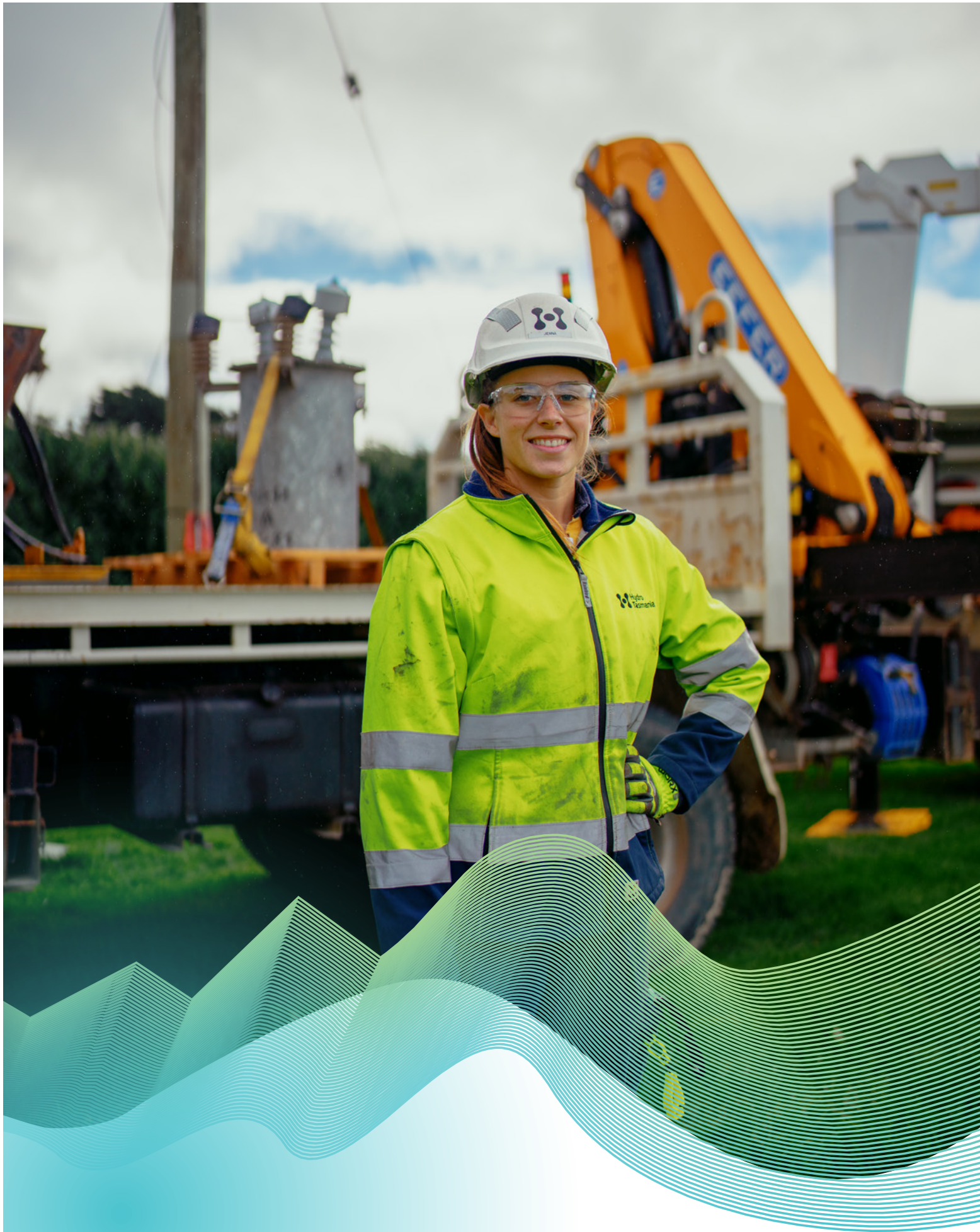
Above: Linesperson Jenna Cook gets ready to do maintenance on a transformer on King Island
