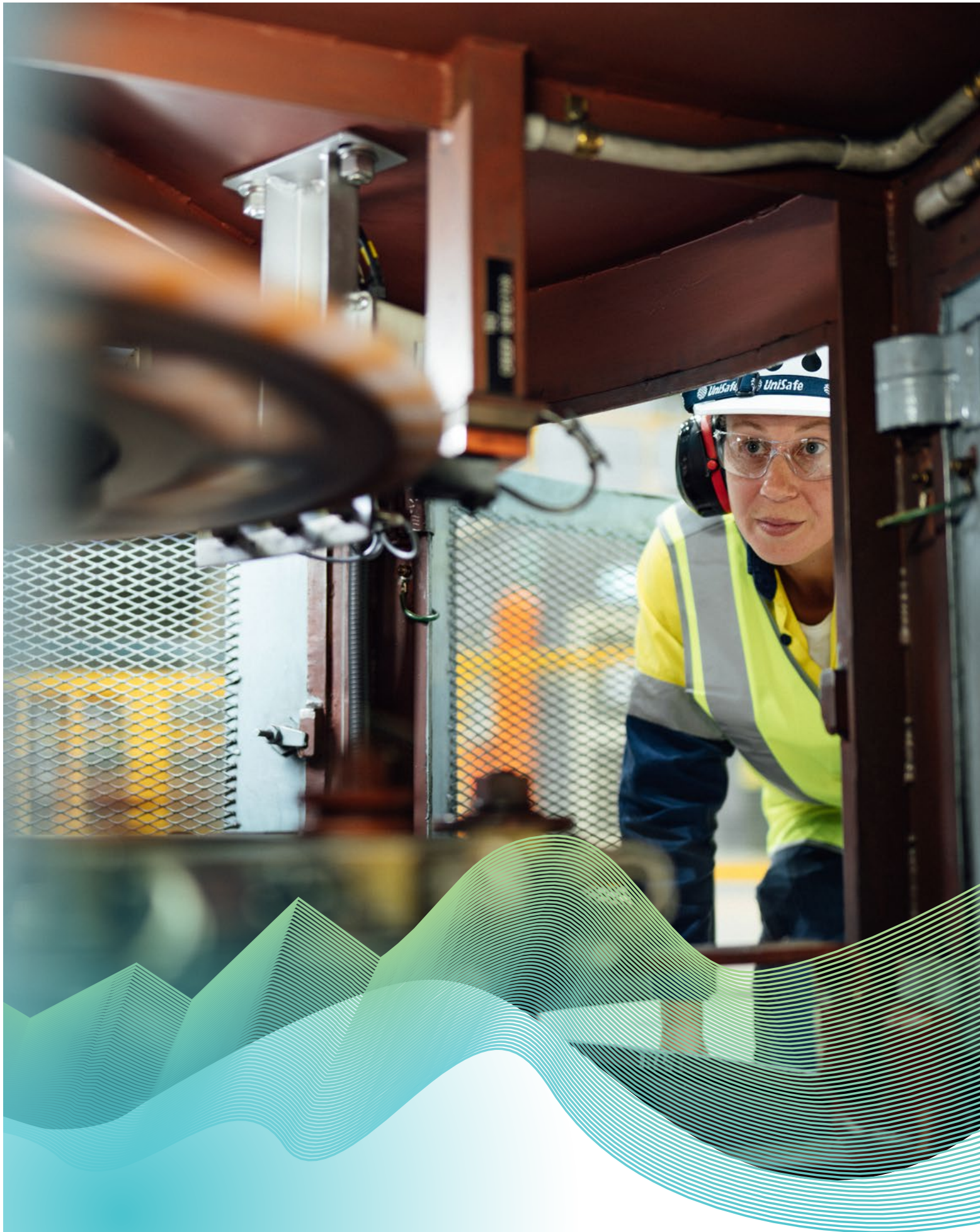
Above: Area Coordinator Leah Powell inspecting a turbine at Mackintosh Power Station
