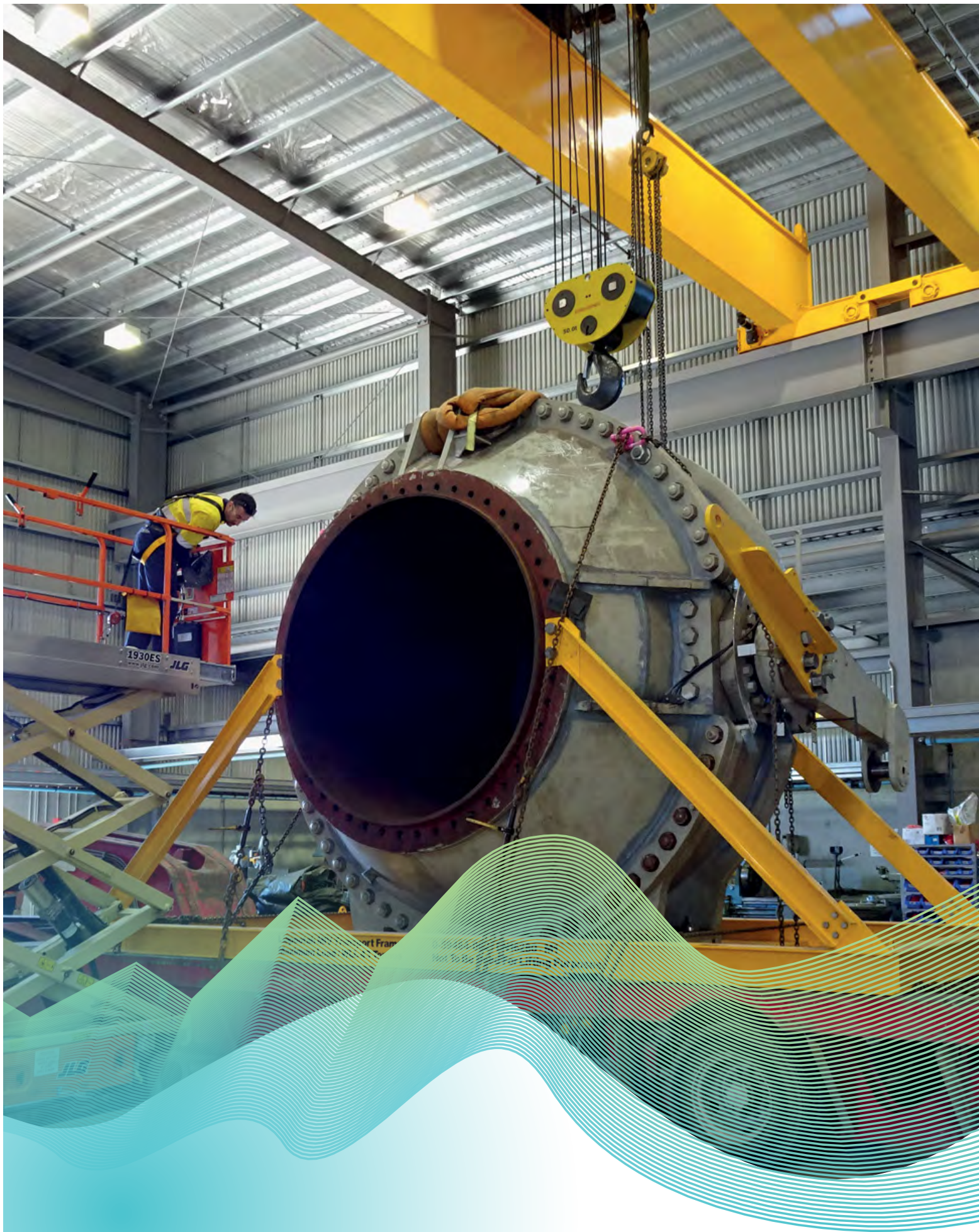
Above: Liapootah no 2 main inlet valve arriving at the Cambridge Workshop for refurbishment
