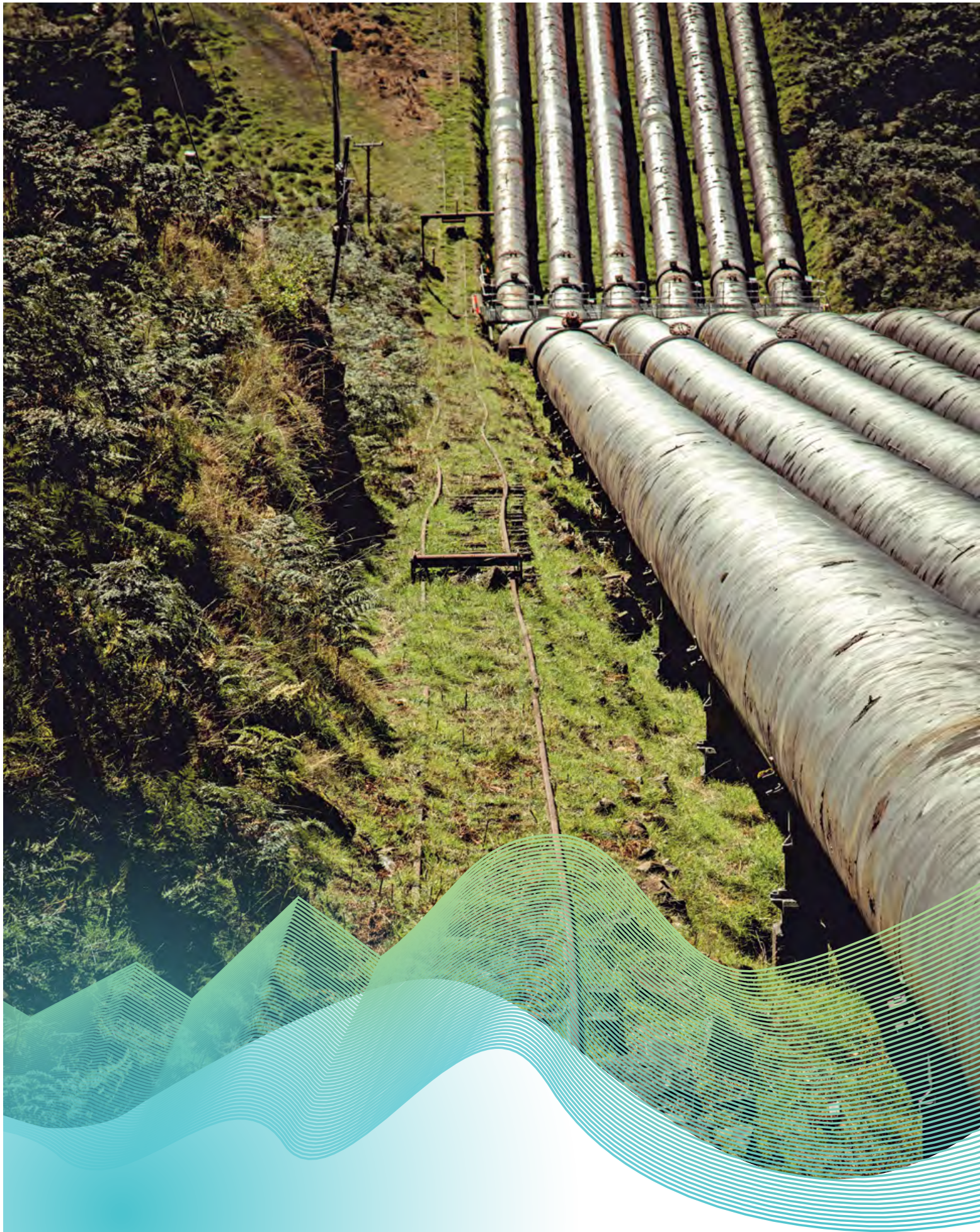
Above: Tarraleah Power Station penstocks
