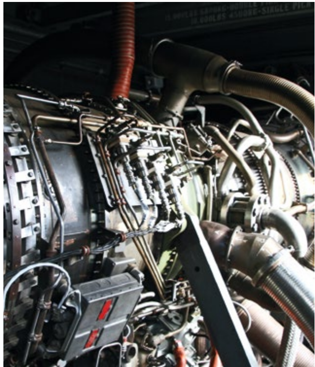
Gas turbine at Tamar Valley Power Station
