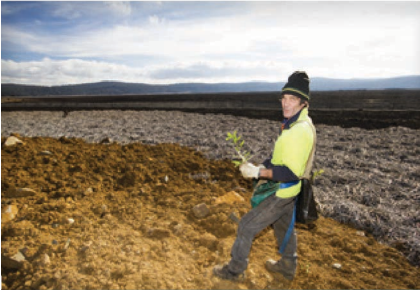
Contractor Graham Harrex conducting rehabilitation work at Lagoon of Islands in central Tasmania
