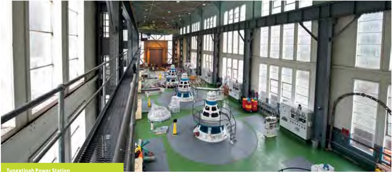
Tungatinah Power Station
