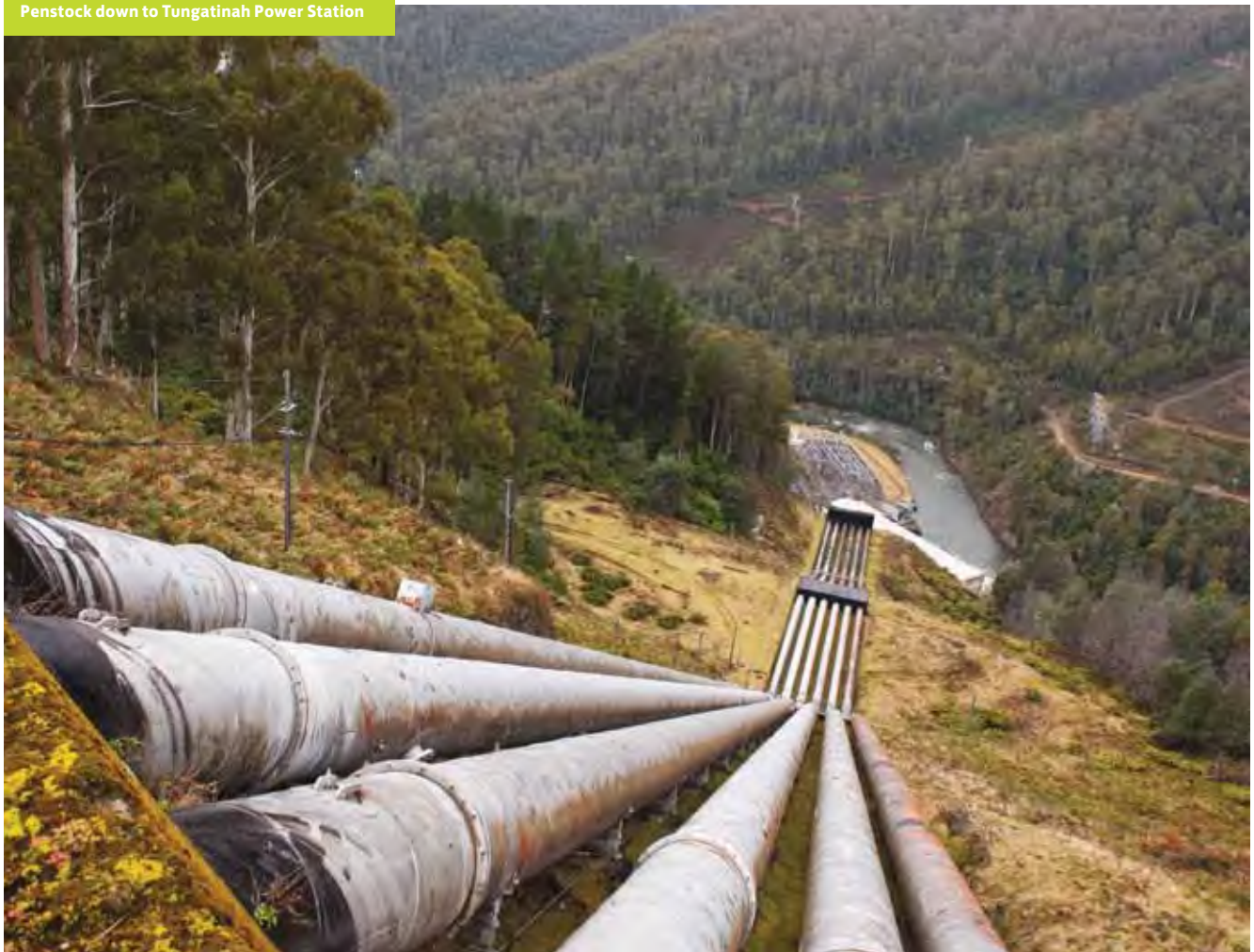
Penstock down to Tungatinah Power Station
