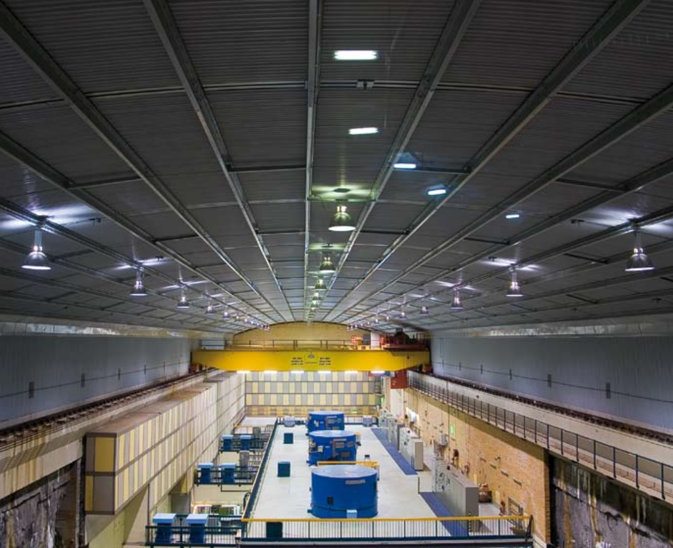
Gordon Power Station
