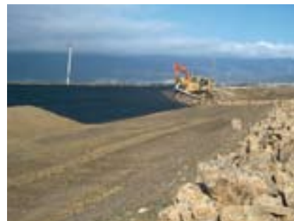
Placement of rip rap and geotextile on banks to eliminate erosion from wave action – Poatina storage
