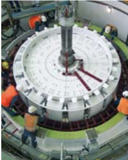
Trevallyn Power Station
