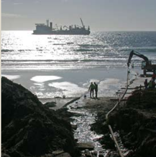
The Basslink cable comes ashore
