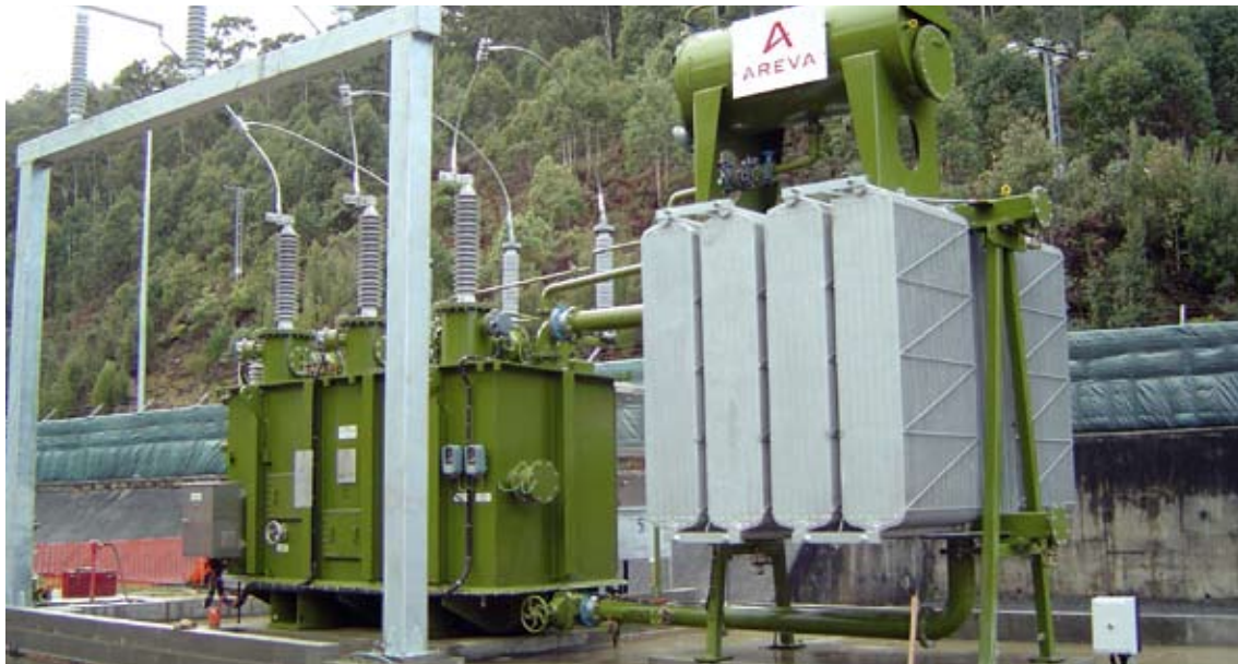
The successfully recommissioned Tungatinah No. 5 transformer
